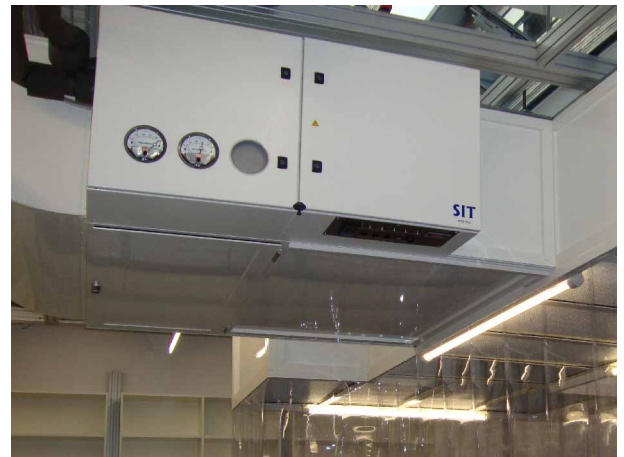
Fig. 2 suspended air handling unit
