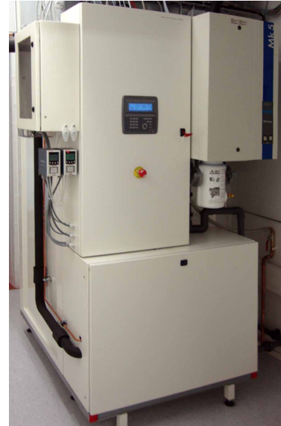
Airhandling units with temperature, humidity, over pressure controller
