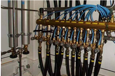
Connection to cooling water, CDA clean dry air
