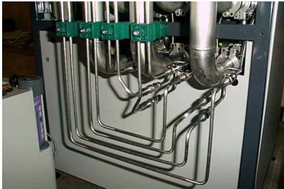
Gas connections, gas abatement systems, scrubbers
